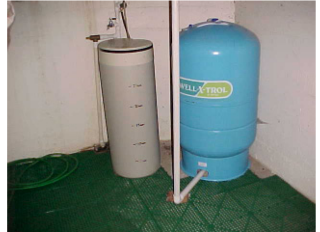
A Hydropneumatic Storage Tank
